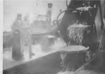
JAN VAN DER VLIES, dredge operator and Jan Hofman, superintendent of the San Nicolas Harbor project for the Royal Netherlands Harbor Works Co., watch the spoil-digging buckets come up from the bottom.
